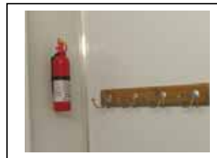
Fire Extinguisher & Coat Hooks
