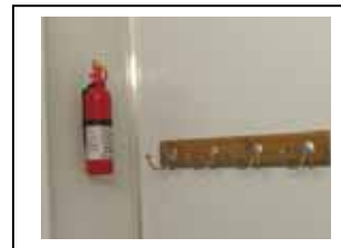
Fire Extinguisher & Coat Hooks
