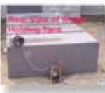
300 Gallon Waste Holding Tank
