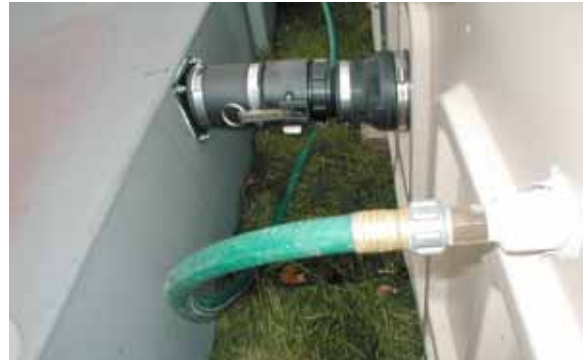
Garden House Hook-Up Holding Tank Hook-Up
