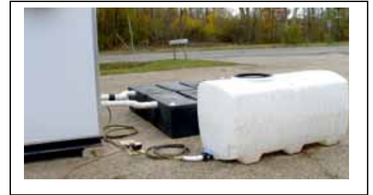
Water Tank and Water Pressure System + Waste Tank Hook-Up
